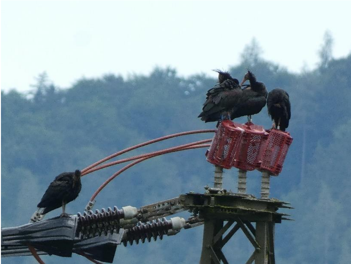
Figure 6. Northern Bald Ibises on a retrofitted power pole in Salzburg. The power pole was secured using cover caps (black), insulation tubes (red), and insulated cages (red). Picture: C. Esterer
