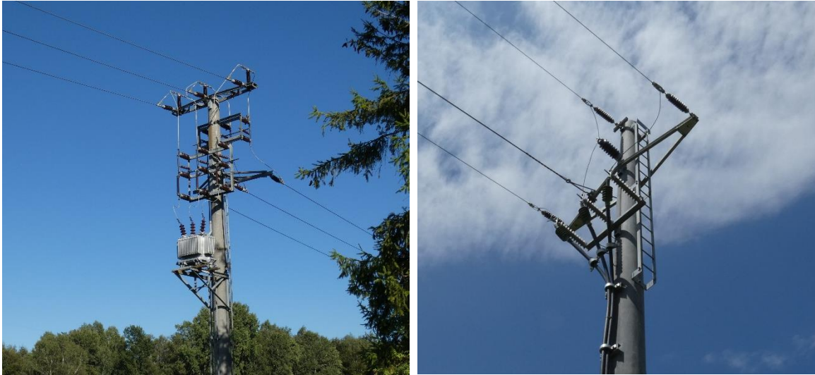
Figure 2a & b. Two high-risk medium-voltage power poles with horizontal insulators and complex constructions in Austria. Pictures: C. Esterer
