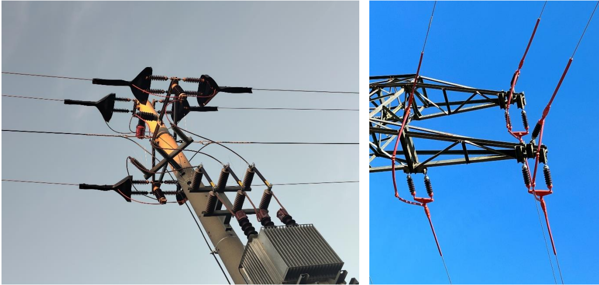
Figure 5. (a, left) Retrofitted power pole in Upper Austria with cover caps (black), insulation tubes (red), and insulated cages (red); (b, right) Retrofitted power pole in Carinthia with insulation tape (red) wrapped around the power line and connection. Pictures: B. Gönner
